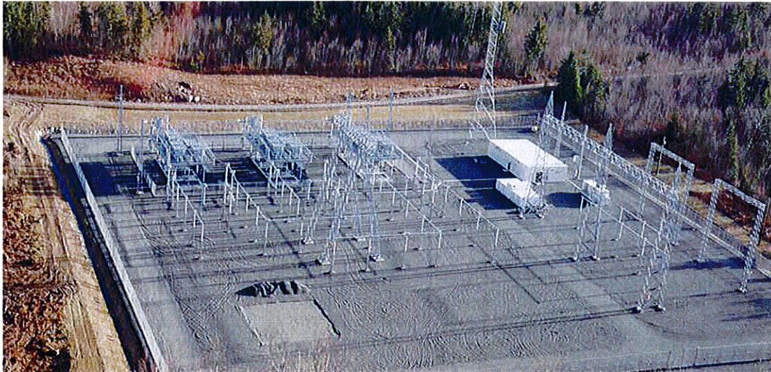
Above: Example of capacitor station at Ruby Creek about 14 kilometers west of Hope.
